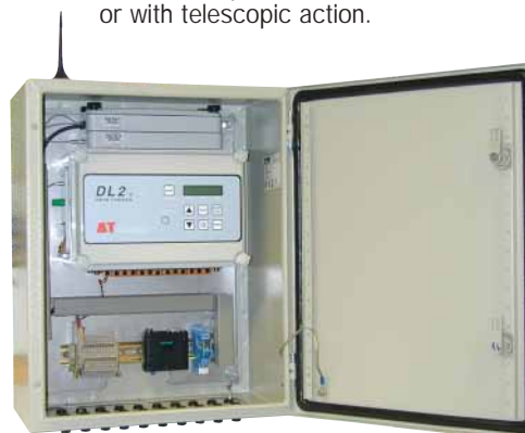
DL2e Logger, GSM modem and antenna, 12V wiring kit and relay, solar power regulator and LBK1 rechargeable battery pack, installed in Weatherproof Enclosure.
