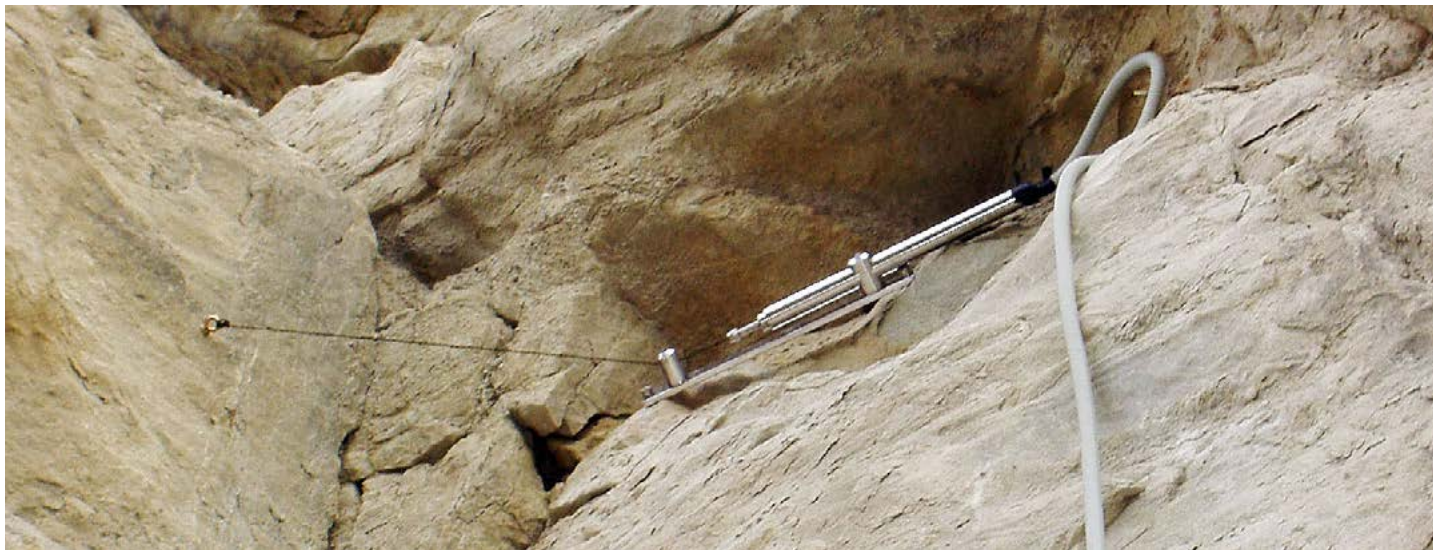
Electrical deformer installed on a rock fall
