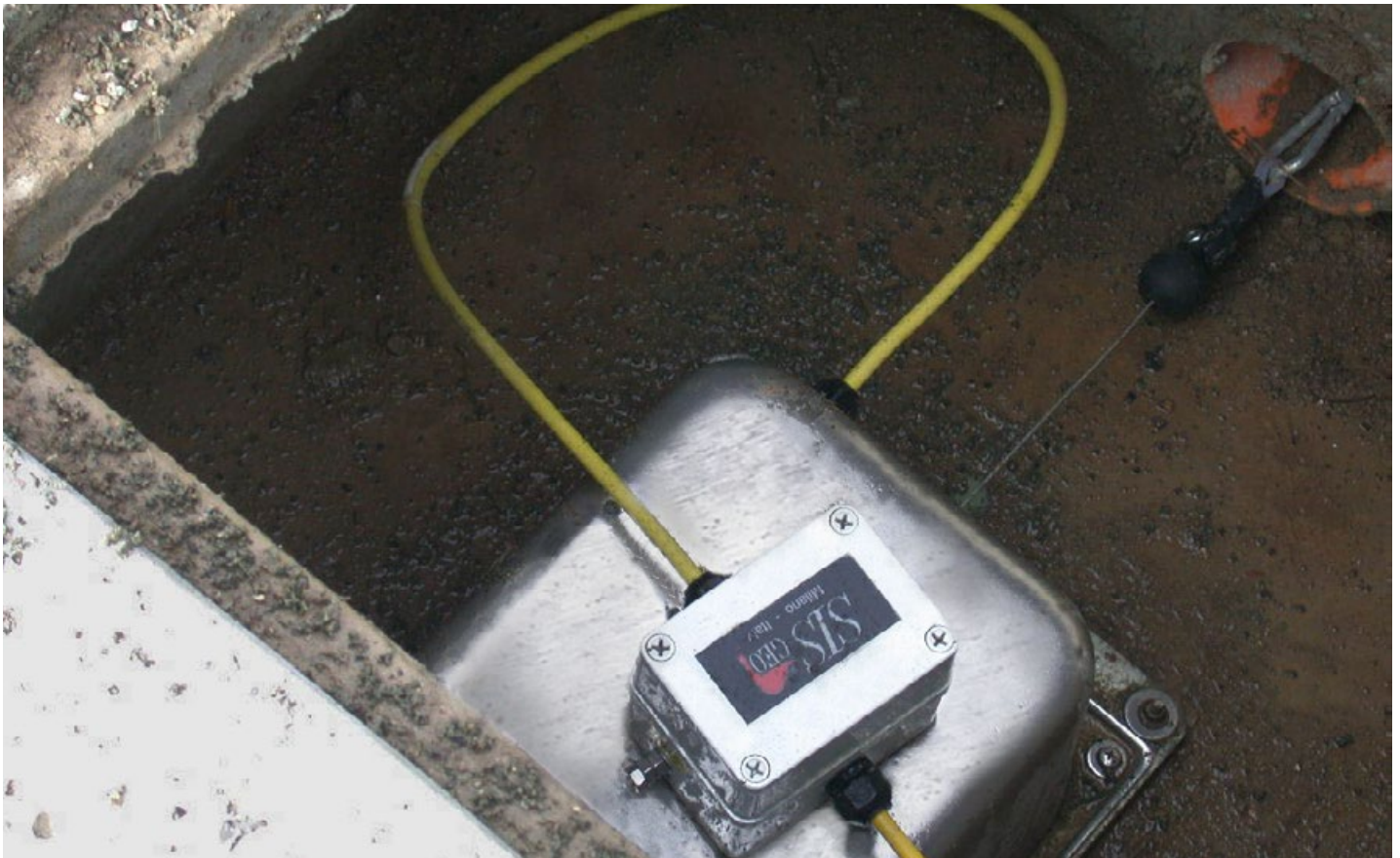
Wire crackmeter installed in a manhole with over voltage protection box
